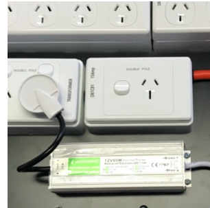
Labeled GPO for transformer
